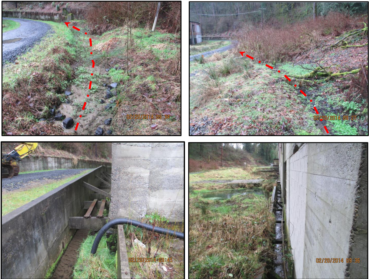
Figure 6. Roadside ditches and open foundation drains that capture and divert water around the east side of the Brewery building complex.
