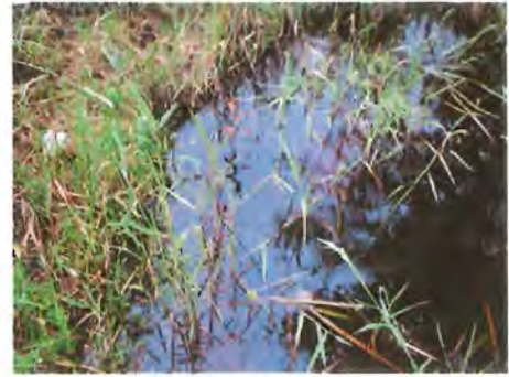
Flooded ditch along 54 th , at Culvert #4
