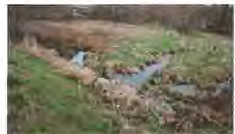
Looking south at 66th Ave. Water back up at Culvert #24, at 66th Ave west of Cavalier Street
