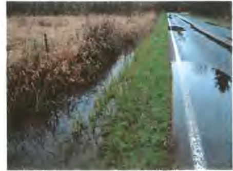
Water entering the roadway from ditch at Kirsop Rd, directly south of 54th
