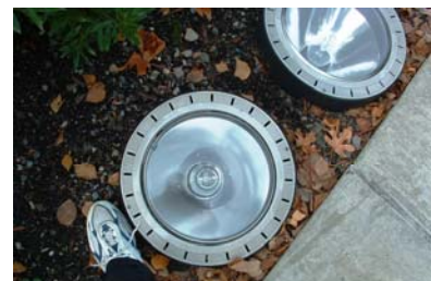
Metal halide flagpole lights DOT Bldg (Linderson Way)
