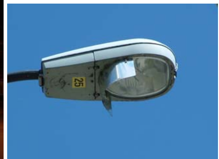
Shield for Streetlight Olympic Way NW (Olympia)
