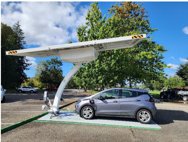
Pilot solar EV charging station installed at Pioneer Park.
