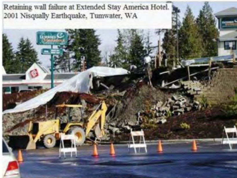
Figure 2: The Extended Stay America facility near the Highway 101/Crosby Boulevard interchange had a large retaining wall give way, which broke a water line (Former Tumwater Fire Chief John Carpenter-phone conversation 6-3/9/10-2009)
