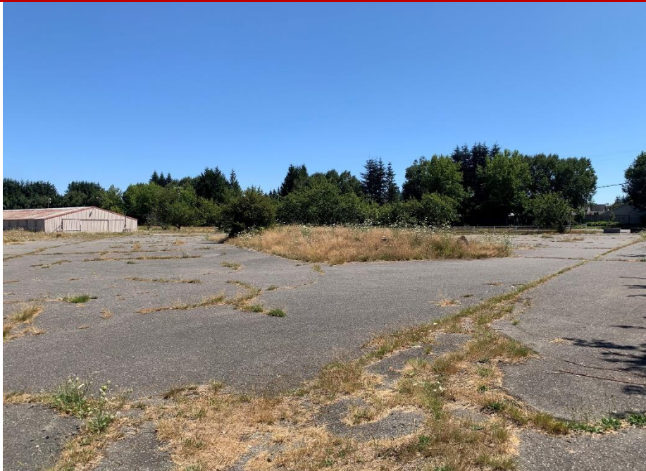
Photo 4: Photo of pavement area taken from the drive entrance on the east side of Trails End Rd SE looking southeast.
