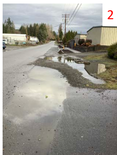
Ponding on Joppa Facing North
