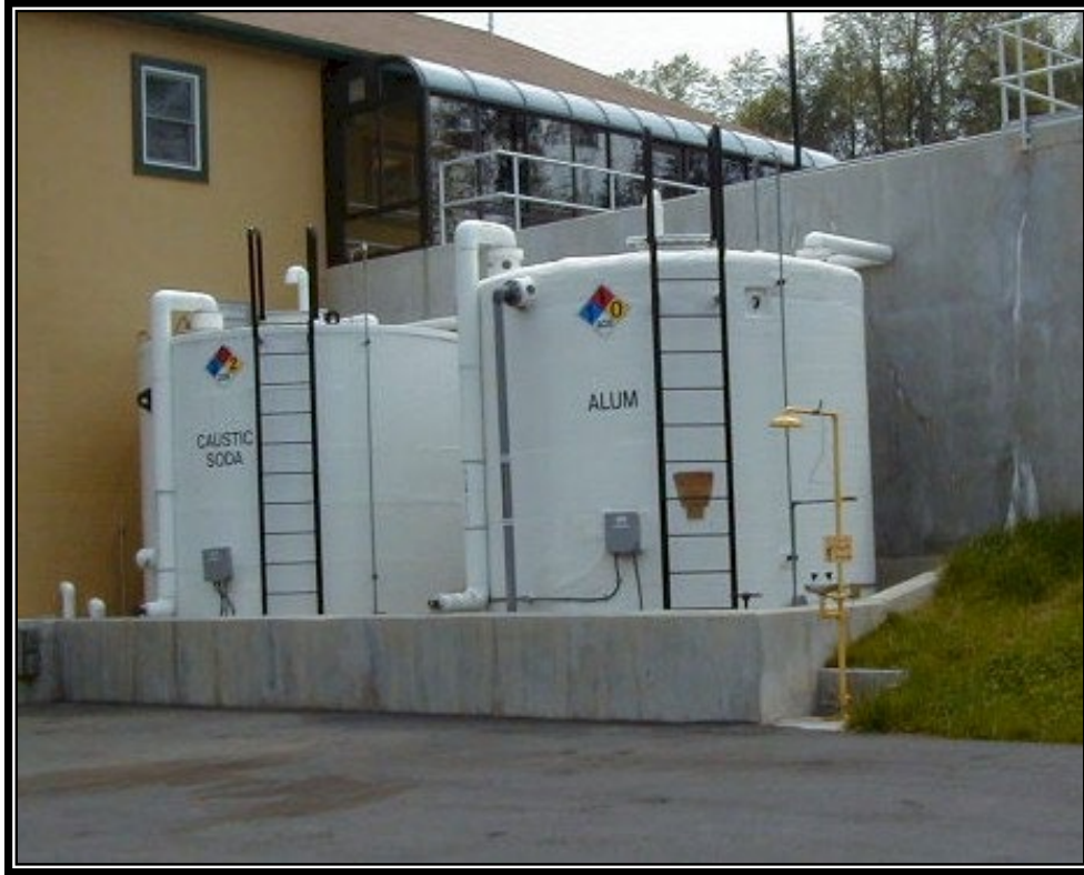
(Photo courtesy of Seattle Public Utilities)
