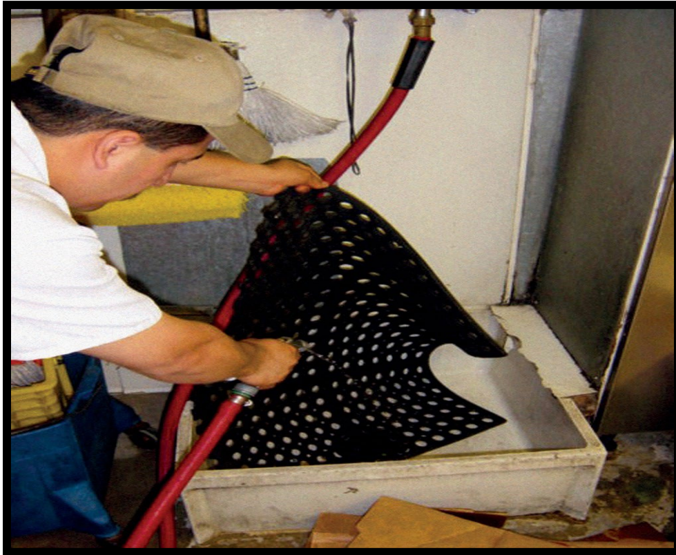
(Photo courtesy of Seattle Public Utilities)
