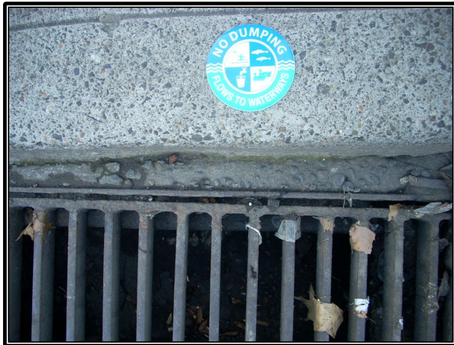
Figure 4.24. “No Dumping” Storm Drain Stencil.
