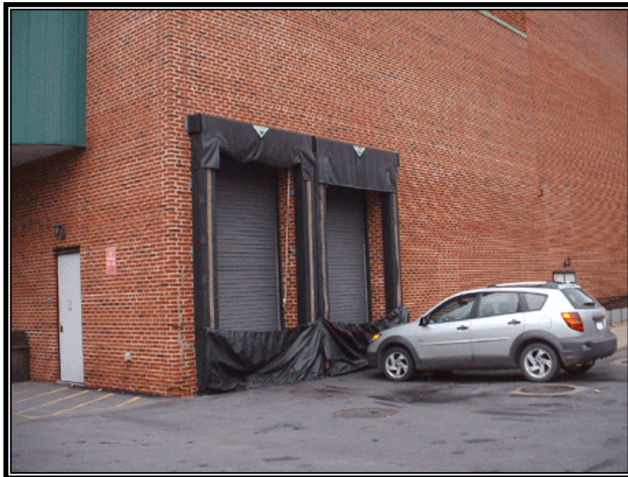
Figure 4.6. Door Skirts to Enclose the Trailer End of a Truck to Prevent Material Contact with Rainwater.
