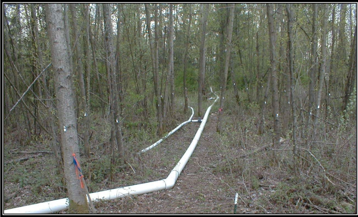
Figure 3.22. Manifold and Branches in a Wooded Vegetative Filtration Area.
