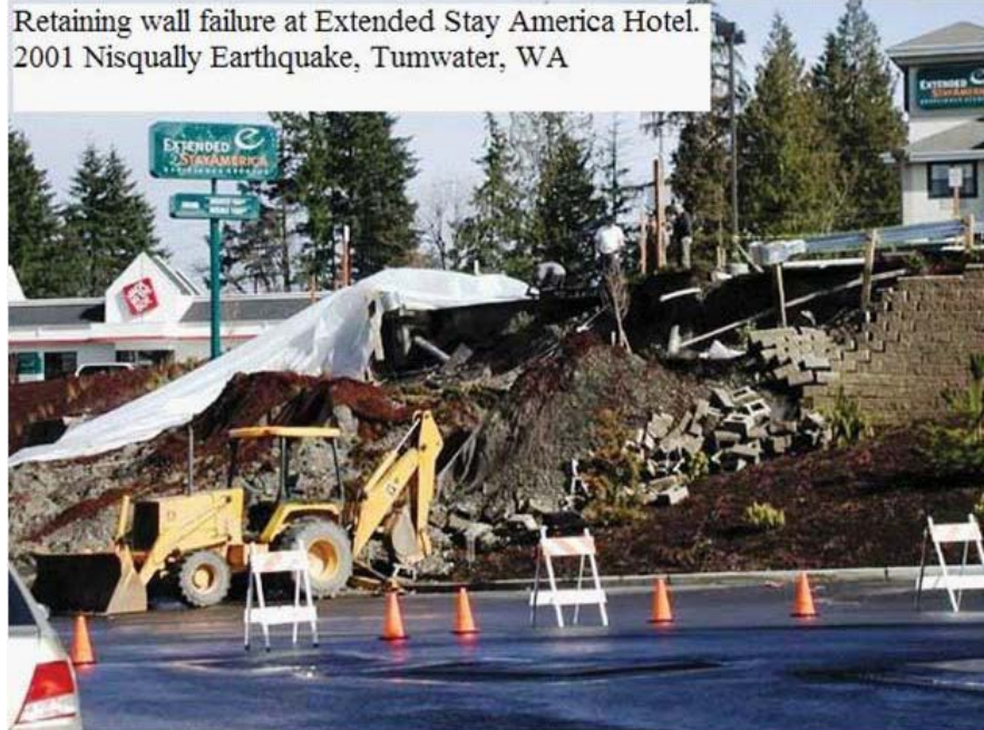
Figure 2: The Extended Stay America facility near the Highway 101/Crosby Boulevard interchange had a large retaining wall give way, which broke a water line (Former Tumwater Fire Chief John Carpenter-phone conversation 6-3/9/10-2009)
