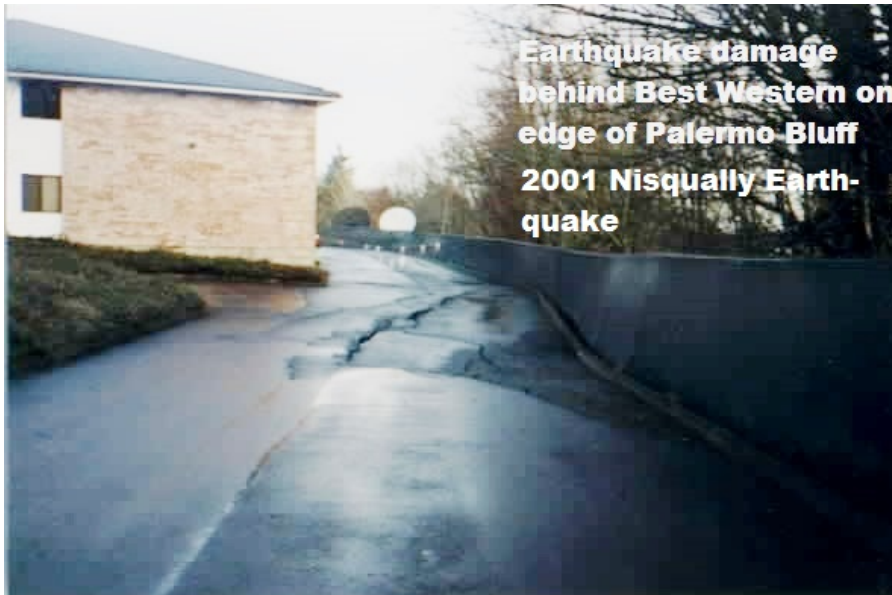
Figure 1: The Best Western hotel located on the bluff above the Palermo well field had a portion of the rear parking lot settle and start to slide down the hill. (Former Tumwater Fire Chief John Carpenter-phone conversation 6-3/9/10-2009)
