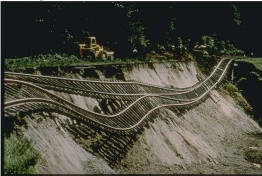
Figure 8-10. Hillside slid away from beneath this four-hundred-foot section of a Union Pacific Railway branch line at Tumwater, near Olympia, Washington, during the Puget Sound Earthquake of 1965. A large landslide during the heavy-rainfall winter of 1996-97 also damaged the rail line. Photo by G.W. Thorsen, Washington Division of Geology and Earth Resources.
