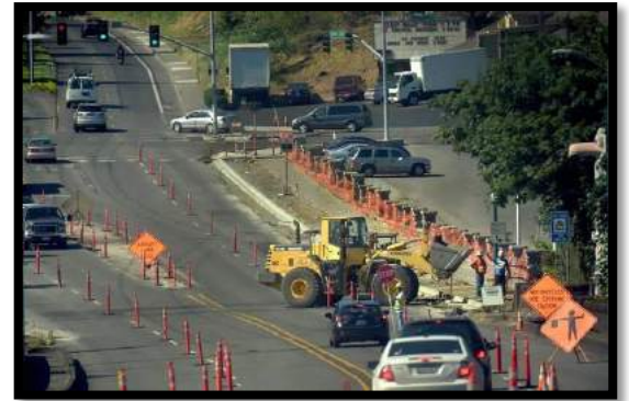
This 2014 Capitol Way project added bike lanes and improved the sidewalks in this part of the Brewery District in addition to improving stormwater runoff facilities.
